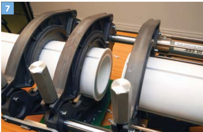
7) Remove the heating plate and quickly inspect the pipe ends for any contaminants before closing the carriage to fuse the joint.
