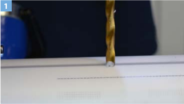
1) Drill the hole in the pipe using a drill bit 1/32" smaller than the repair plug.
